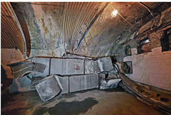
Plant room in the wartime BBC section of Clifton Rocks railway, showing applied corrugated sheeting to keep masonry falls from damaging machinery, and also some fallen ventilation ductwork. The wall at the right hand side is the external wall visible from Portway Road
